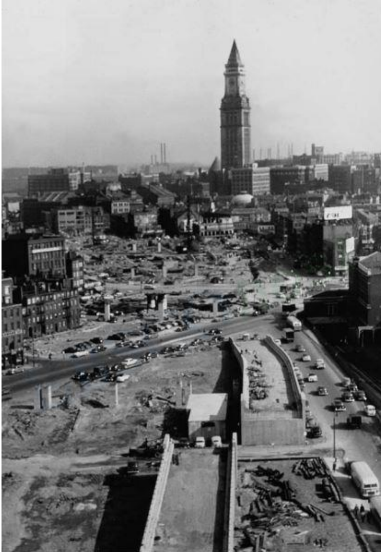
The first Central Artery being built in Boston in the late 1950's. The existing buildings in its path were demolished. Accessed from Boston Public Library, Print Department; photograph by Leslie Jones.
